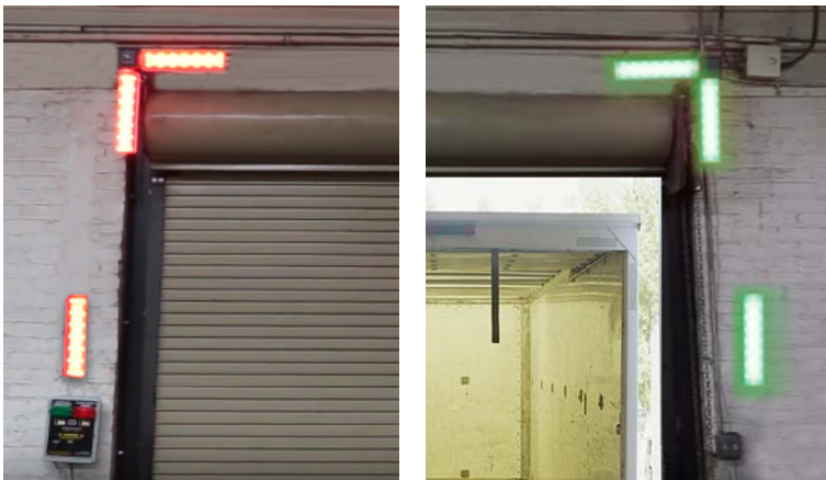
TopDok turns from red to green when a loading vehicle is properly restrained.
